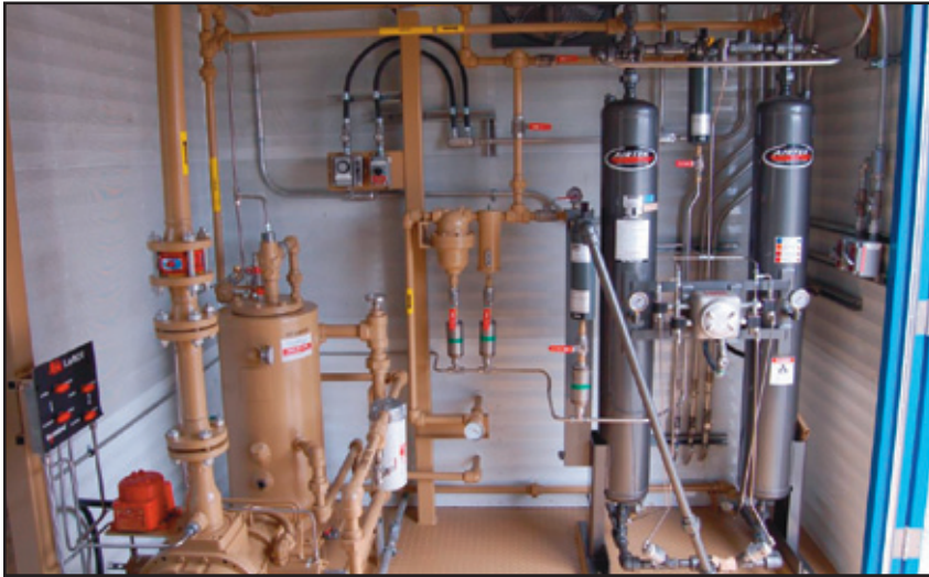
Included in the package for Delphi Automotive is a twin-tower self-regenerating gas dryer. When one tower is being used to dehydrate the gas stream to the testing facility, the other tower is regenerating itself by having a slipstream of compressed gas flow over the desiccant bed to remove the water. The towers change functions on a fixed time cycle. The saturated natural gas is fed into the suction side of the compressor.
